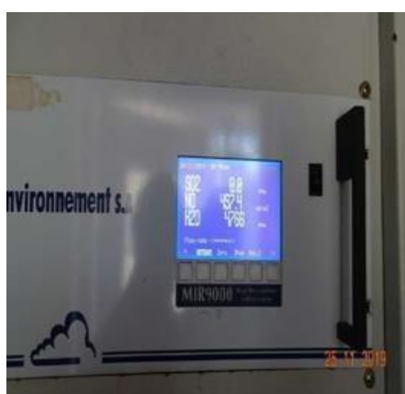
Continuous Emission Monitoring System Panel
